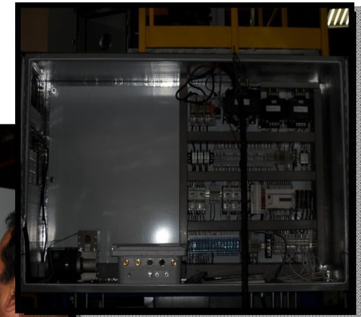
Inside control panel
